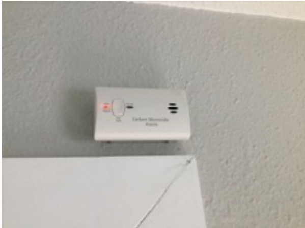
Carbon Monoxide Detector Installed
