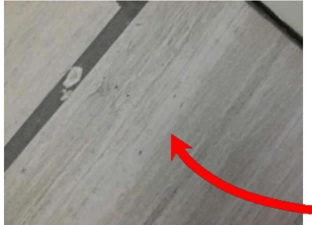
Flooring - Discolored grout
