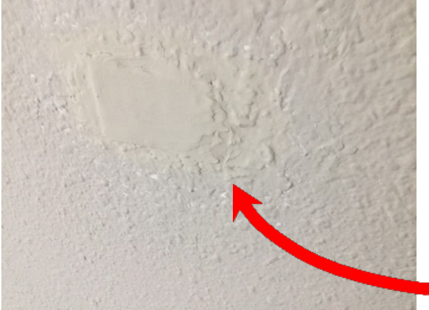
Walls/Paint - Non matching repair and touch up.
