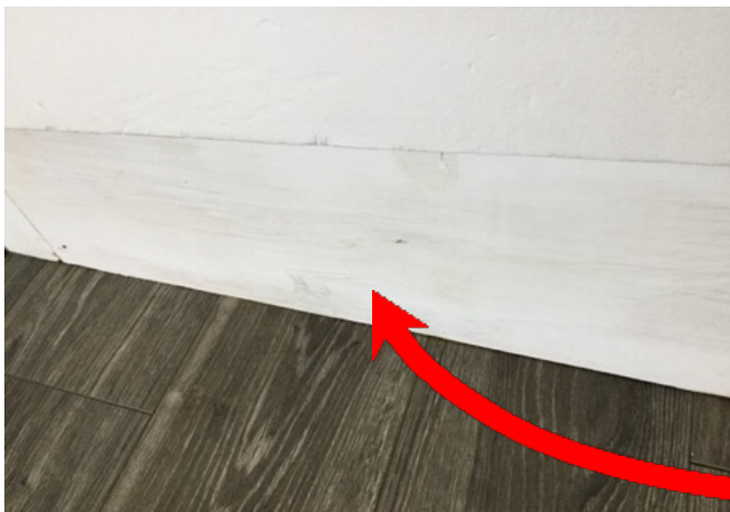
Bedroom 1 Closets Bleed through on paint at bottom of door
