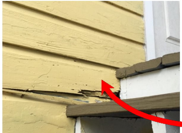
Walls/Siding/Trim - Rotted siding
