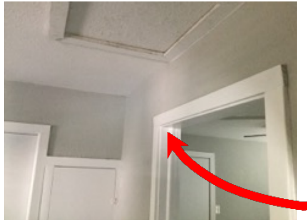
Smoke Alarm Removed - MISSING: smoke alarm as required by code.
