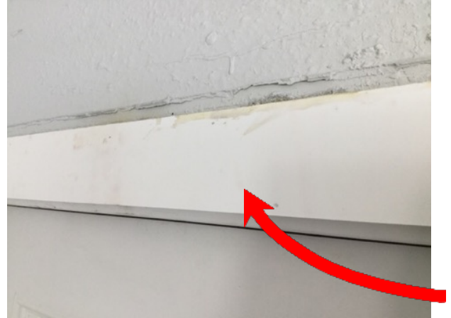
Front Door Interior - Discolored doorframe
