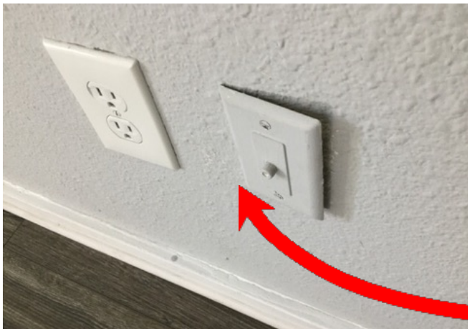
Bedroom 1 Outlet/Switch Covers Not flush with wall
