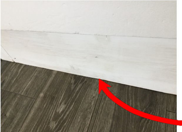
Closets - Bleed through on paint at bottom of door
