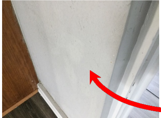
Walls/Paint - Non matching touch up and discolored wall
