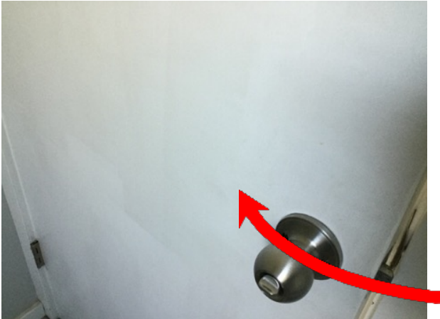
Door - Excessive bleed through on paint
