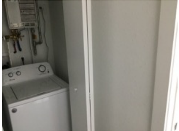
Carbon Monoxide Detector Missing
