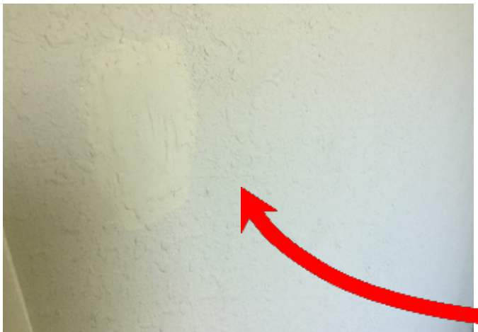
Bathroom 1 Walls/Paint Non matching touch up
