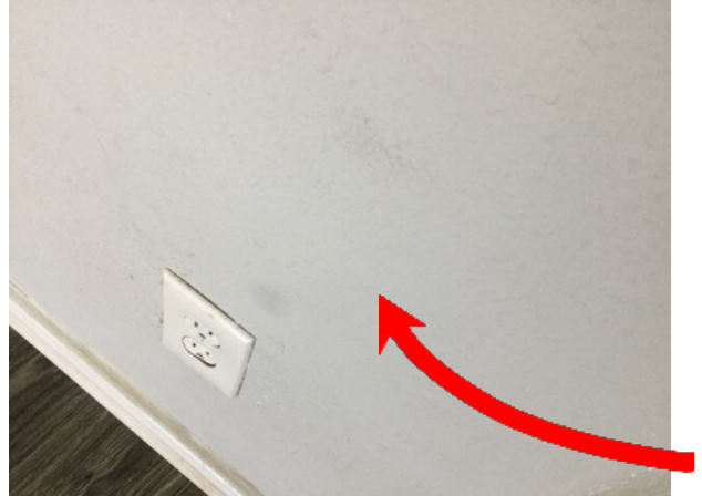
Walls/Paint - The wall is discolored
