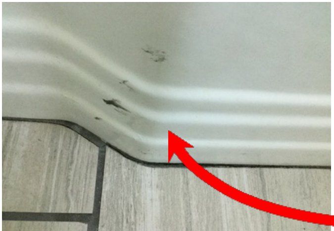
Bathroom 1 Tub/Fixture Marks on outside of tub
