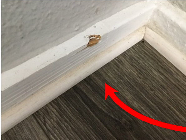
Baseboards - Damaged and discolored
