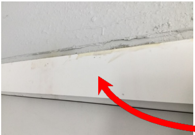
Entry Front Door Interior Discolored doorframe
