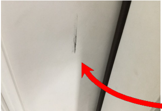
Entry Front Door Interior Scuffs on door.
