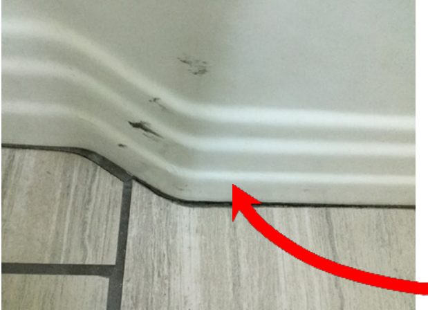
Tub/Fixture - Marks on outside of tub
