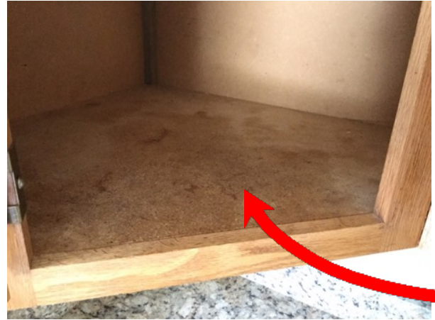
Upper Cabinets - Stained inside base
