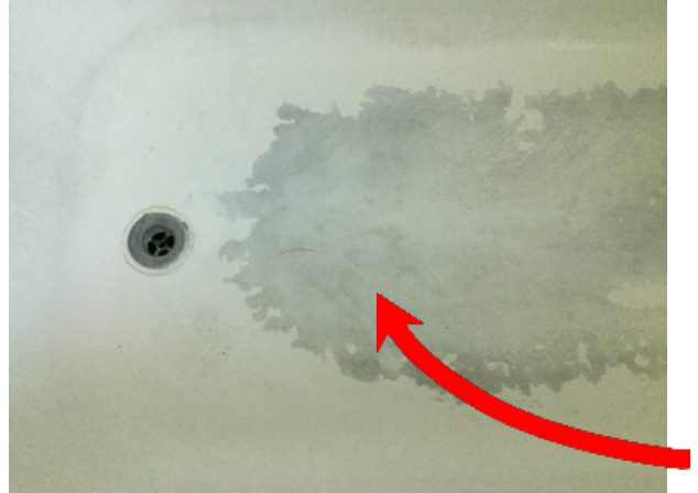
Tub/Fixture - Peeling paint. The floor is discolored around the base of the tub.
