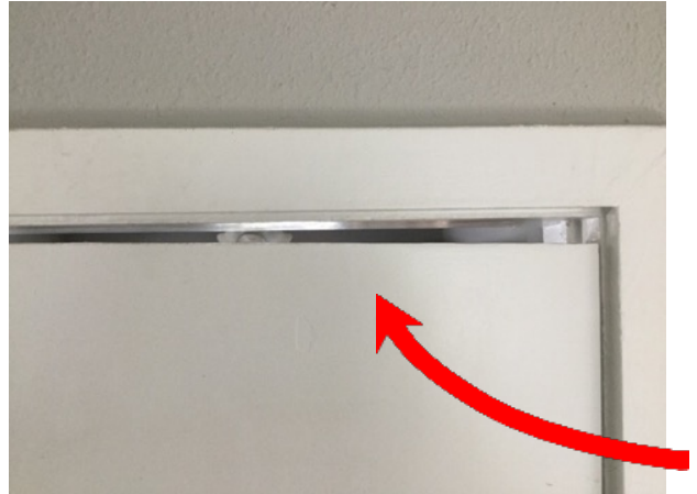
Door - Large gap between door and doorframe at top of door
