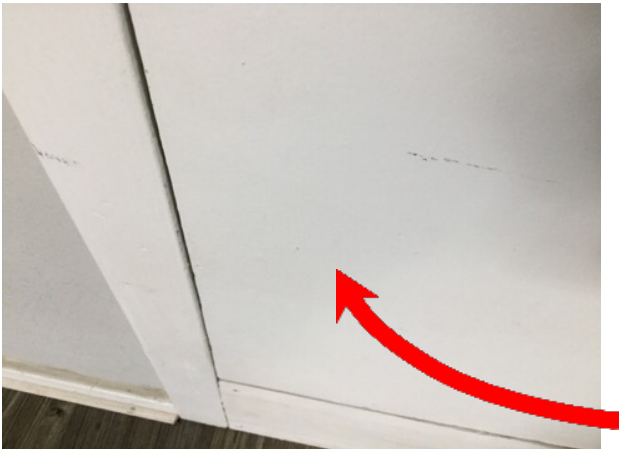
Closets - Scuffs on door
