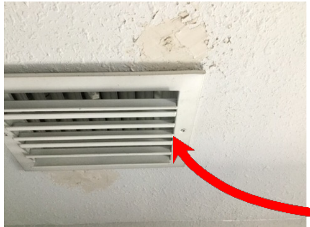
Ceiling - Unfinished discolored repairs The ceiling is discolored.
