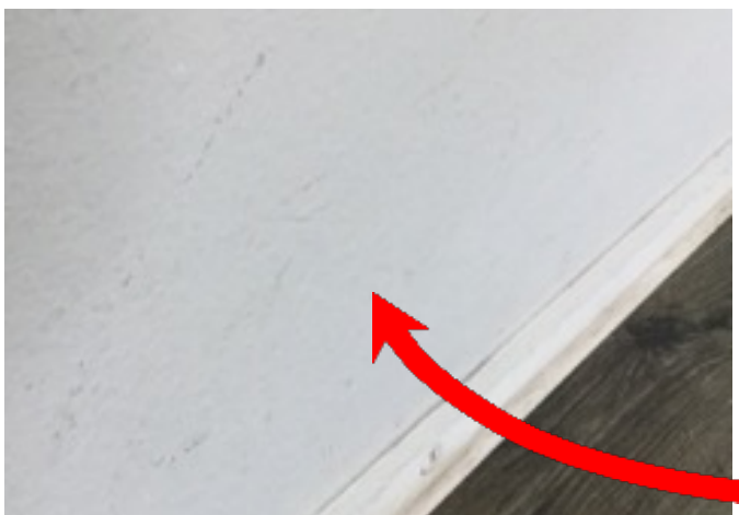
Living Room Walls/Paint The wall is discolored
