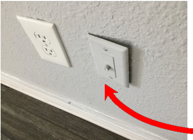
Outlet/Switch Covers - Not flush with wall
