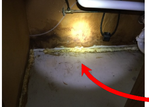
Cabinet Under Sink - The base of the cabinet is discolored. Sunken base
