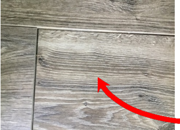
Flooring - Gap in flooring
