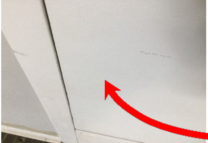
Bedroom 1 Closets Scuffs on door
