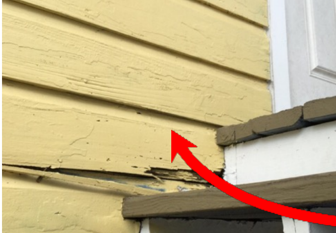
Front Exterior Walls/Siding/Trim Rotted siding
