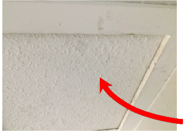
Ceiling - The ceiling is discolored.
