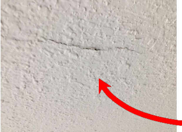
Ceiling - Cracks in ceiling.
