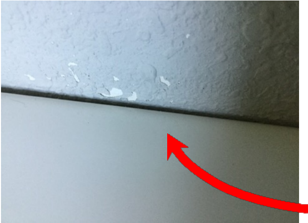
Walls/Paint - Peeling paint
