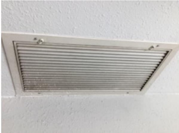
AC Filter - FILTER CONDITION: Filter clogged: Dirt/hair/lint/ etc.
