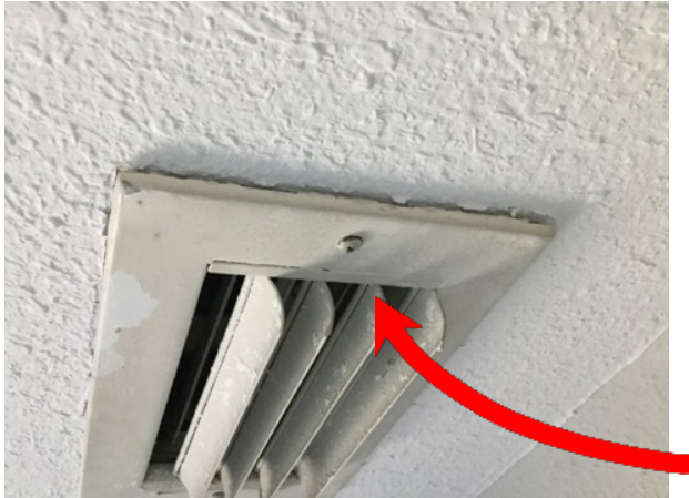
AC Vent - Not screwed tight up against ceiling
