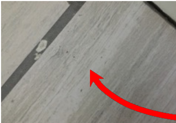
Bathroom 1 Flooring Discolored grout
