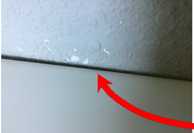
Bathroom 1 Walls/Paint Peeling paint
