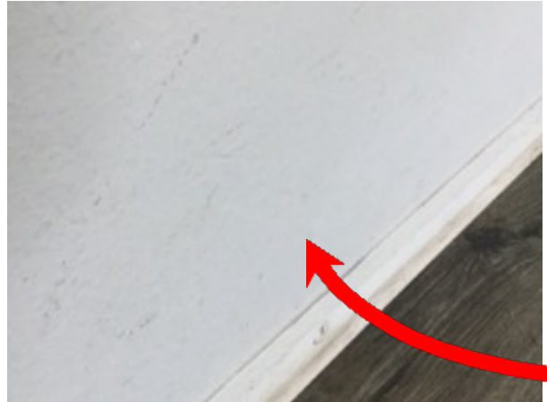
Walls/Paint - The wall is discolored
