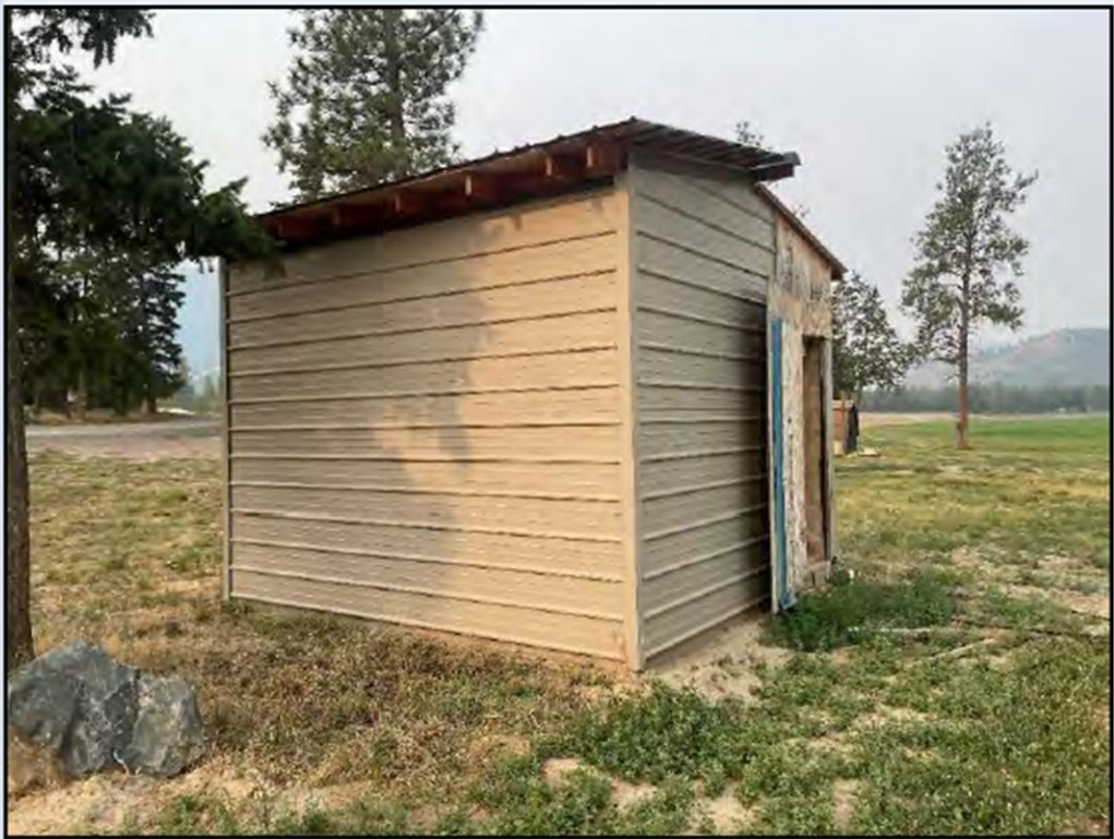
Potable water pump house
