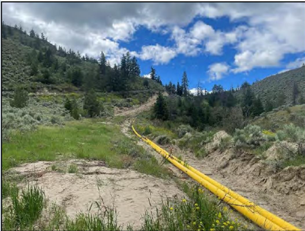
Water supply lines from pump house
